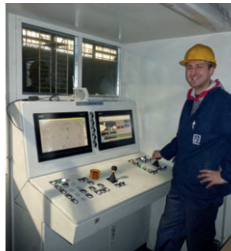
Operator control desk of pouring furnace
